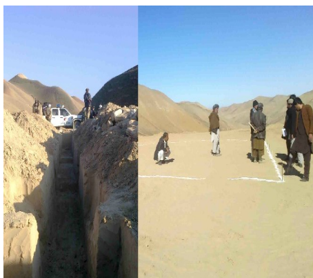
Construction of Ganda basic health centre in Sayad district of Saripul province
