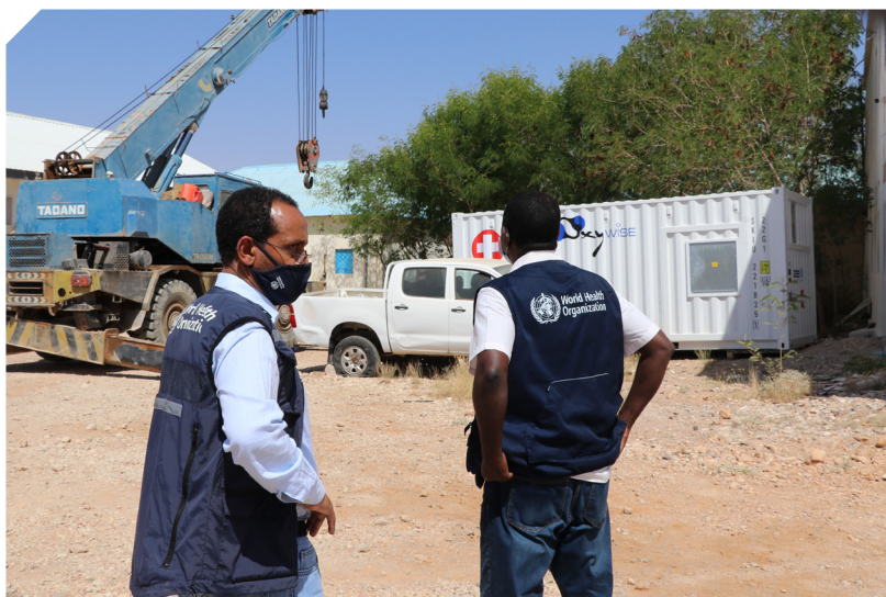
WHO and the Ministry of Health begin the installation of an oxygen plant in Puntland @WHO
