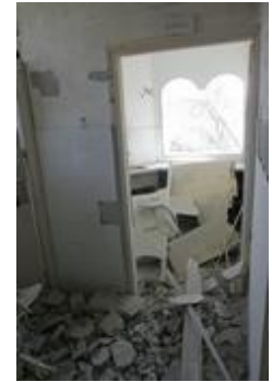
The heavily damaged, al Zanna clinic, operated by the MoH in Khan Younis.
