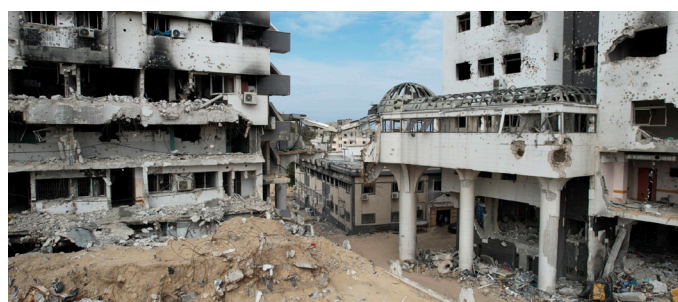
Al-Shifa Hospital, which was severely destroyed after attacks and raid. © WHO
