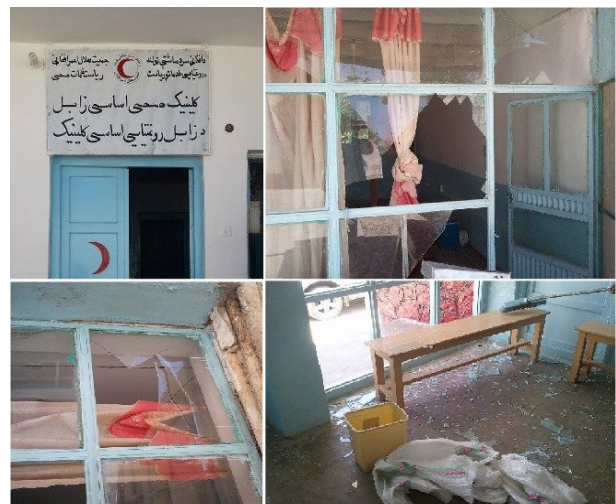
The doors and windows of Zabul Basic Health Centre in Qalat City run by ARCS were destroyed by an explosion
