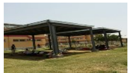
Trusses constructed by WHO in Kunduz Regional hospital to provide triaging space
