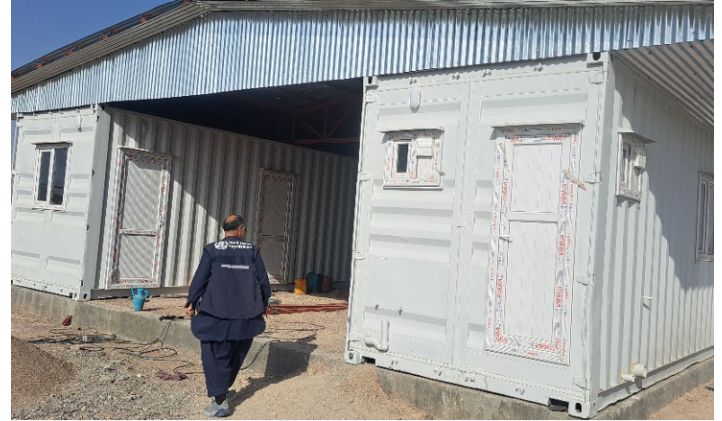
In collaboration with OCCD, WHO is working on the establishment of eight SHCs with containers in the earthquake-affected areas.
