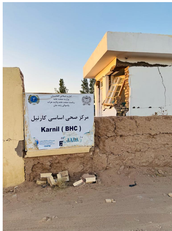
Karnil BHC, located in Zindajan district, which covers almost 15,000 population has been completely destroyed.
