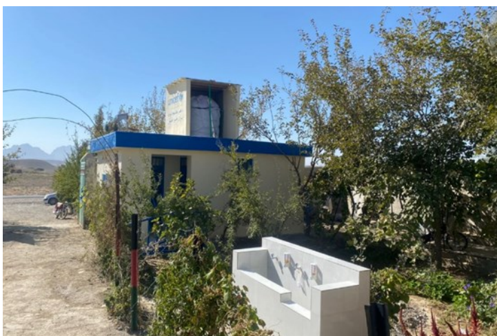
Figure 4. Construction of safe water facility in a health care center, Zabul province, Afghanistan, October 2022
